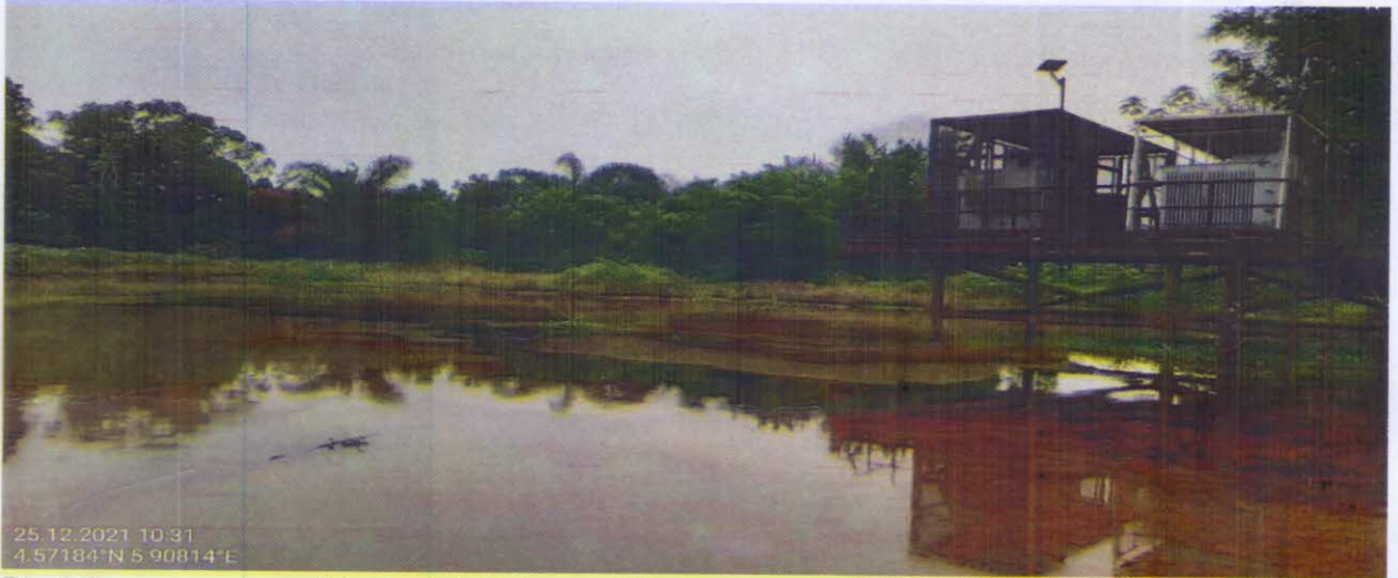
Pic 1.2 Electronic Submersible Pump not Functioning
